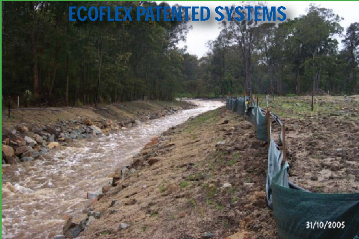
Scour Protection Mats, Malabar Creek, Moruya, NSW
